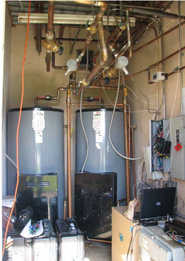
Figure 1-3. Lake Towers Installation
